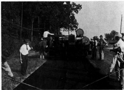
Figure 5. Placing Type F-1 Surface Containing Reclaimed Rubber with Adnun Paver - Note absence of "pulling" in uncompact material.
