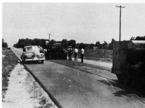
Figure 4. Placing Type F-1 Surface Containing Natural Rubber with Barber-Greene Paver - Note slight "pulling" of uncompact surface. Picture shows completed westbound lane and eastbound lane where binder course has not been applied.
