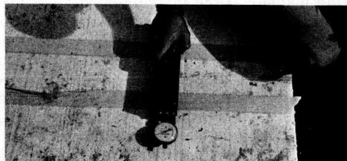
Figure 47. Measuring crack opening with Whittemore strain gage.
