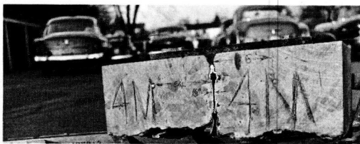
Figure 4. Condition of joint filler in expansion joints 1M, 3M and 4M. The original filler was 1/2 in. thick. In the above joints it measures 1/8 in. in joints 1M and 4M and 1/4 in. in joint 3M.
