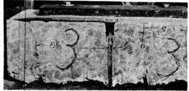
Figure 10. Expansion joint filler originally 3/4 in. non-extruding fiber filler. It now measures 1/2 in.
