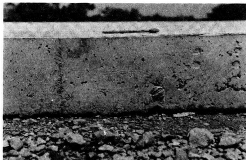
Figure 5. Edge view of typical crack at the age of 10 days (Falls-McLennan County Project).
