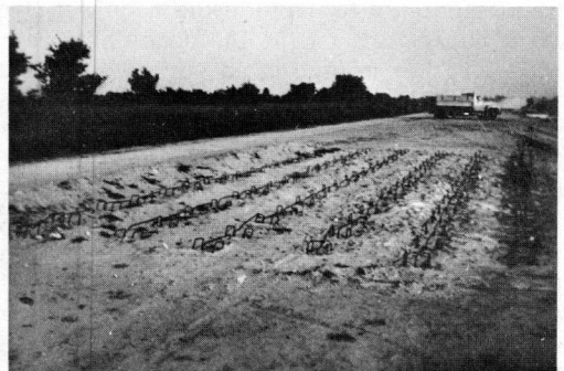
Figure 2. Test Road between Zwartberg and Meeuwen, Belgium: One of the abutments—fins poured and reinforcements placed. Slab will have to be poured afterwards.
