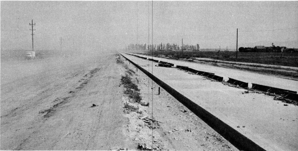
Figure 5. Typical dust formation on untreated sections 5 hours after cessation of watering operations. Wind speed 20-25 mph. Note reduced visibility on existing travelway on left side of photograph. Median had previously been heavily watered for more than a month and tightly compacted by movement of water trucks.
