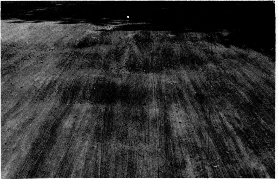
Figure 2. Road surface with washboard formations developed.
