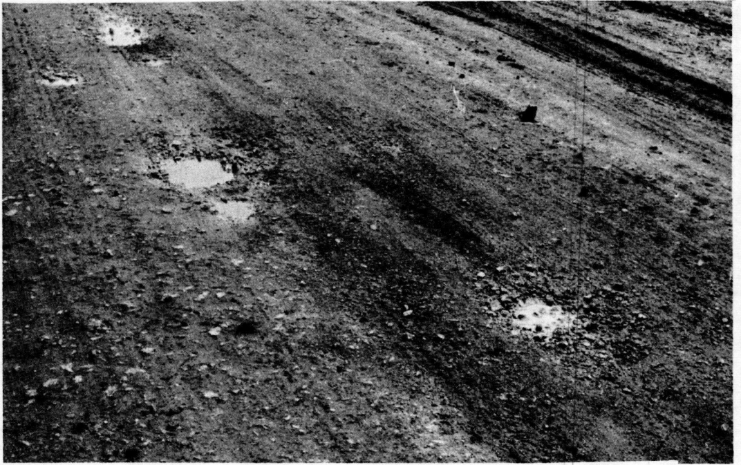
Figure 1. Typical potholed road surface.
