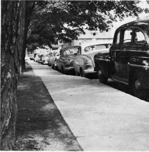
Figure 1. Uneven settlement of sidewalk caused by removal of soil moisture by large trees.
