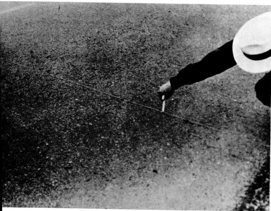
Fig. 3. Station 460+00, \frac{1}{4} -in. rutting in outer wheel path of traffic lane, eastbound roadway, August 16, 1960.
