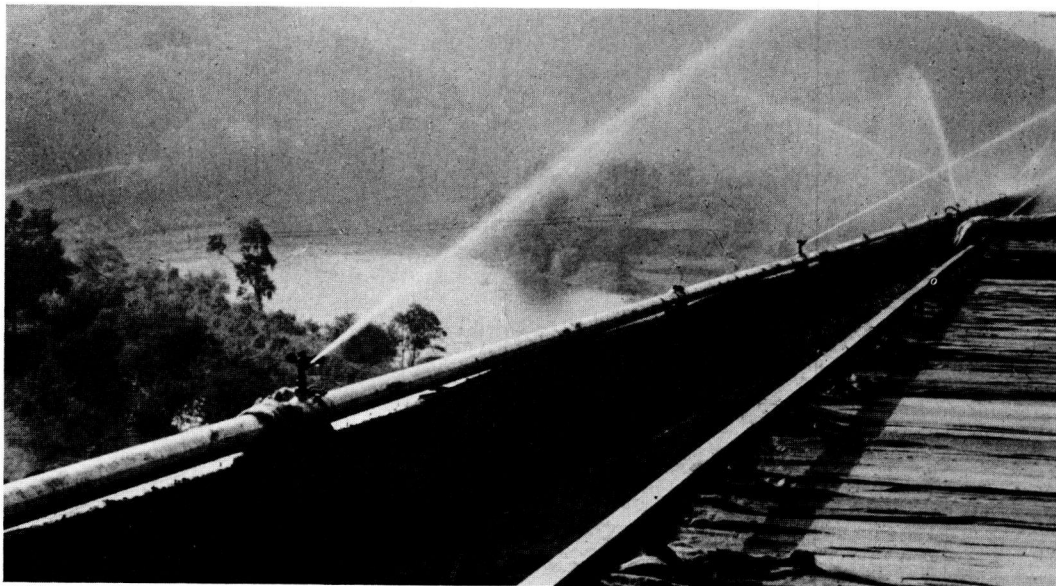
Figure 10. When wet burlap is used for curing it must be kept saturated.
