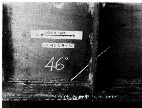
Figure 15. Web crack at type C stiffener (intermittent web weld).
