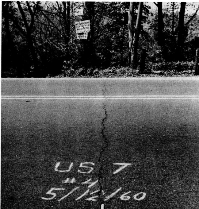
Figure 4. Uncontrolled Joint Crack Project No. 1—Route US 7, Norwalk, May 12, 1960.
