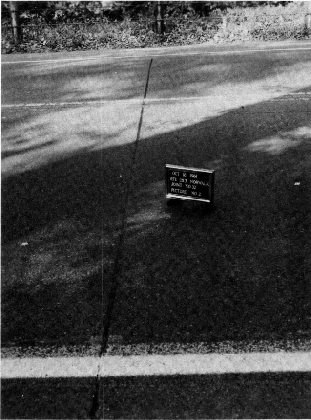
Figure 5. Controlled Joint Crack Project No. 1—Route US 7, Norwalk, October 18, 1961.
