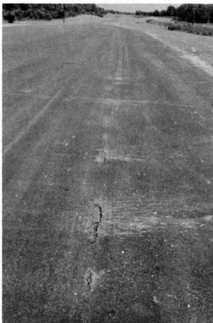
Figure 7. Same area as shown in Figures 5 and 6. A double crack over edge of fabric nearest outside edge of pavement has permitted water and dust to seep in; traffic passing over cracks has splashed water and dust onto surrounding pavement discoloring it.
