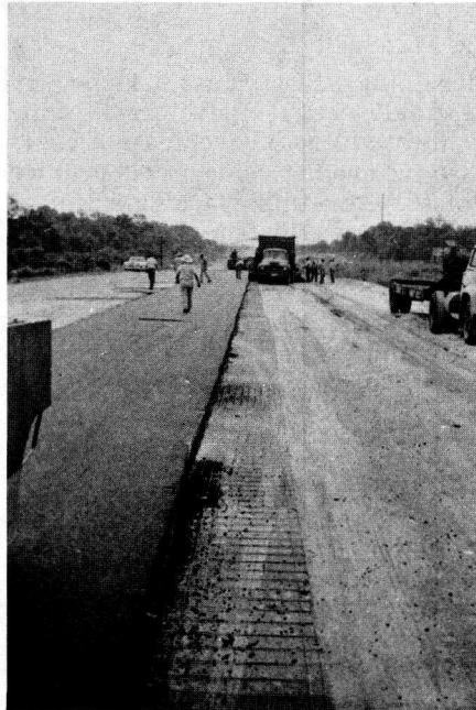
Figure 6. Same strip of fabric (Fig. 5) after surface course has been placed over one-half of it. Practically all bulges have been removed by crimping; evidence of cracking in the fresh surface course seen near exposed fabric in foreground. Note end of strip protruding through the surface course in center of photograph.
