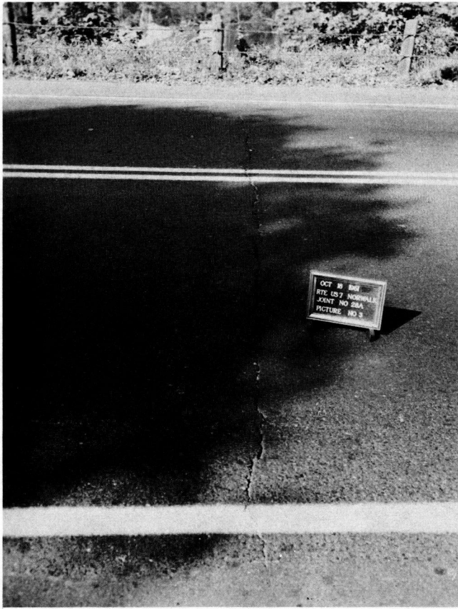
Figure 6. Uncontrolled Joint Crack Project No. 1—Route US 7, Norwalk, October 18, 1961.
