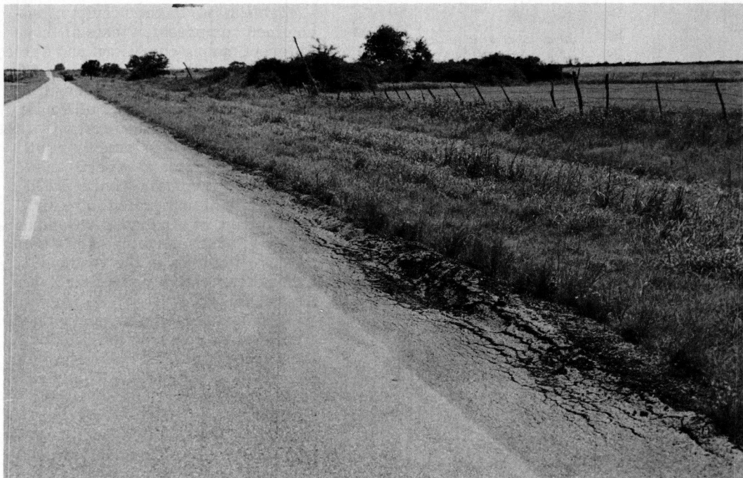
Figure 13. Typical edge failure on test section before reconstruction.
