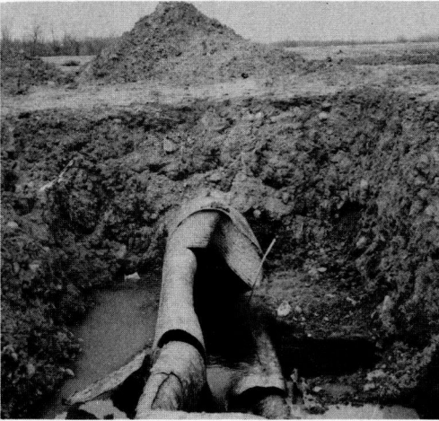
Figure 24. Failure of 96-in. 8 ga. corrugated metal pipe.
