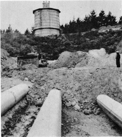
Figure 5. (a) Initial spreading of backfill with D4 loader. (b) progressive back-filling around deep pipe with pneumatic compacting; and (c) leveling backfill over deep fill with 1-ft fill (pipes in foreground are access tunnels).
