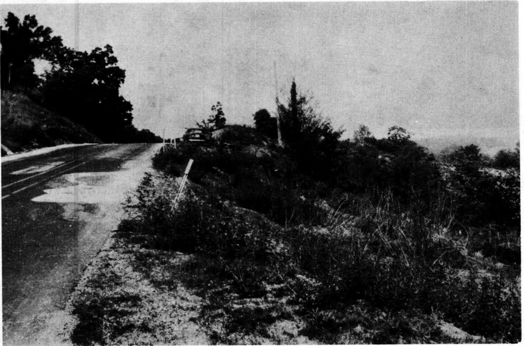
Figure 3. Landslide on Indiana Route 62. Movement of the embankment undercuts pavement in the right lane.
