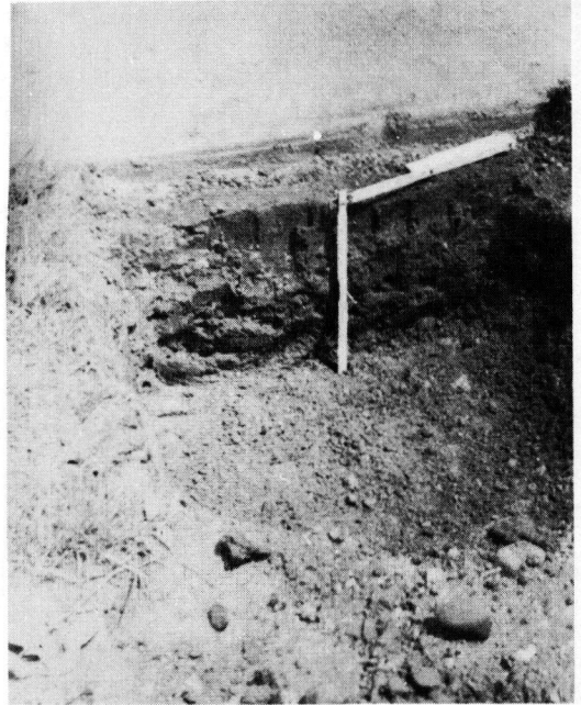
Figure 6. Beginning of investigation at an edge-blow (second-stage) near Station 260+33 of Project 13 D2 on US 40. At this stage a hole has been opened to the top of the subgrade treatment course leaving the vertical granular wall filling the edge-blow cavity and a clay dam in place. Note the top of the granular wall along the pavement edge and the dry condition of the granular material in the bottom of the hole.
