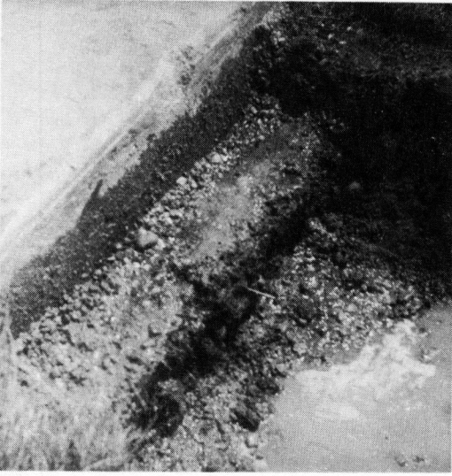
Figure 7. A continuation of the investigation at Station 260+33. At this stage part of the clay dam and granular wall filling the cavity has been removed allowing the water to drain from under the pavement. Note opening under pavement edge where water flowing from beneath the pavement has broken the wall of granular material.
