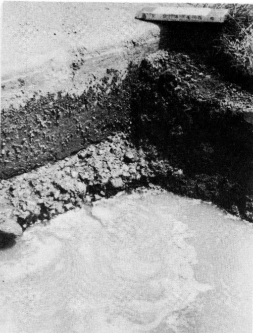
Figure 8. Final stage of the investigation at Station 260+33. Note the cavities under the pavement edge and the continuation of the granular material along the edge of pavement beyond the limits of the excavation.
