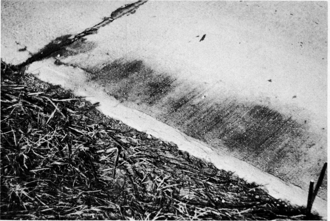
Figure B. Edge condition near Station 260+33 on Project 13 D2 18 months after an edge-blow was excavated and backfilled. Replacement and compaction of shoulder material have removed conditions causing the edge-blow illustrated in Figures 6, 7 and 8.
