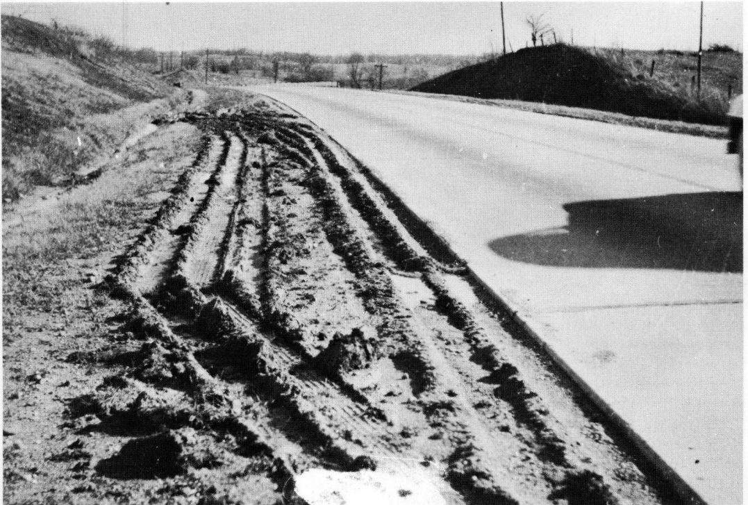
Figure A. Shoulder condition where edge-blows were associated with poor maintenance.
