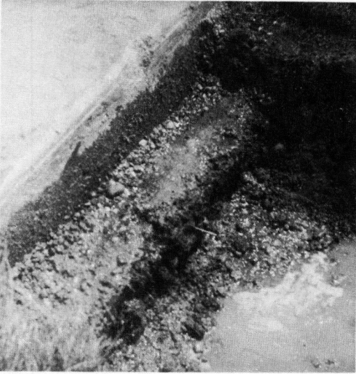
Figure 7. A continuation of the investigation at Station 260+33. At this stage part of the clay dam and granular wall filling the cavity has been removed allowing the water to drain from under the pavement. Note opening under pavement edge where water flowing from beneath the pavement has broken the wall of granular material.
