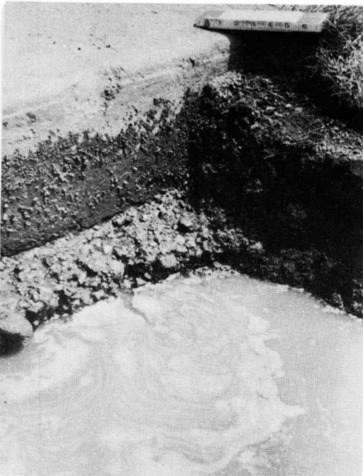
Figure 8. Final stage of the investigation at Station 260+33. Note the cavities under the pavement edge and the continuation of the granular material along the edge of pavement beyond the limits of the excavation.
