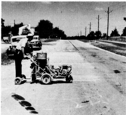
Figure 1. 1950 Transverse stripe location. Stripes on bituminous surface are immediately behind striper and on concrete surface in the background.
