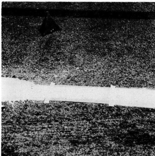
Figure 2. Application-rate determination; 1-ft. strip of kraft paper is shown in place after striping machine has passed over it.
