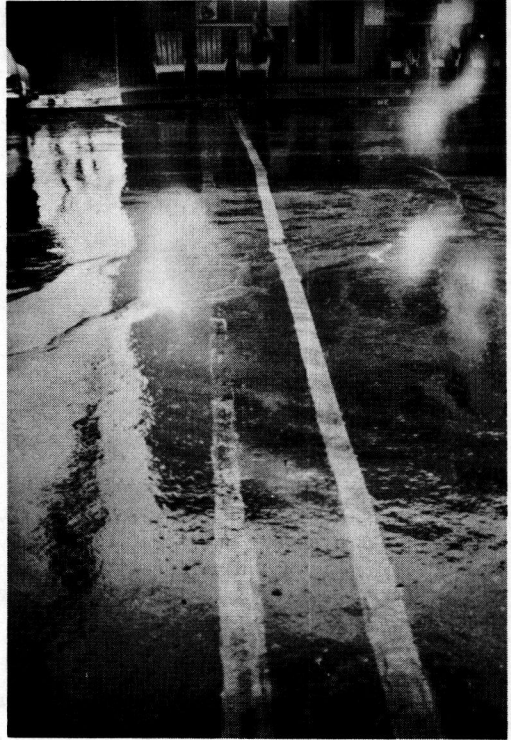
Figure 3. Stripes shown in Figure 2 after 5 months' service. Paint stripe was repainted twice.
