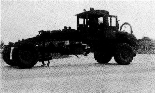
Figure 12. A power patrol used by one of the contractors for longitudinal joint cutting and cleaning.
