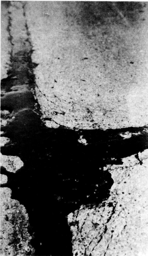
Figure 1. Development of cracking adjacent to a joint intersection.
