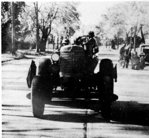
Figure 8. Tractor equipped with a special cutter, hydraulically controlled by operator. This machine is in operation, cleaning, roughening, and refacing longitudinal joints in Duluth, Minnesota. It can also be used for transverse joints.
