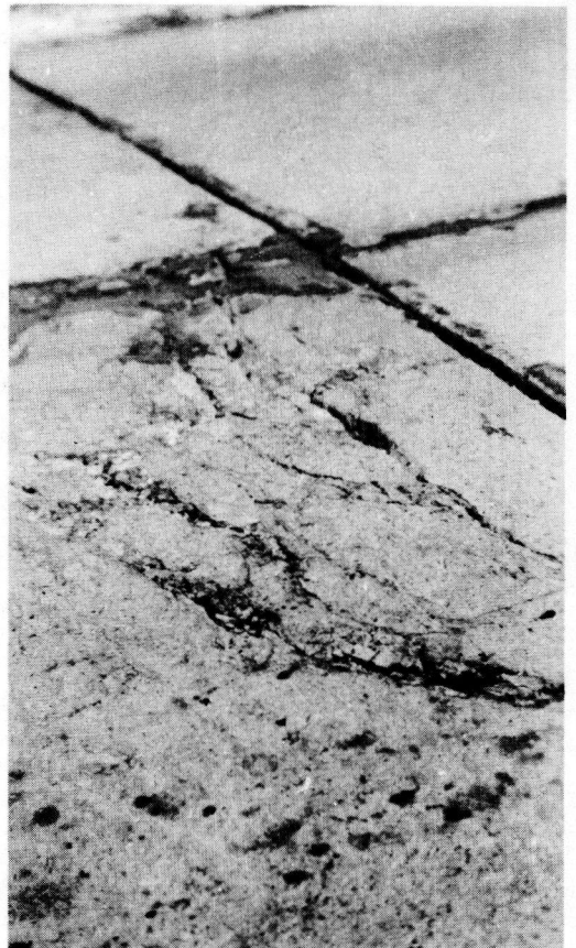
Figure 2. Advanced stage of deterioration at a joint intersection.
