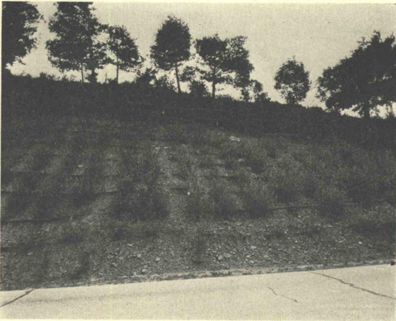
Figure 6. White willow posts and logs to protect slope three months after planting, Pennsylvania.
