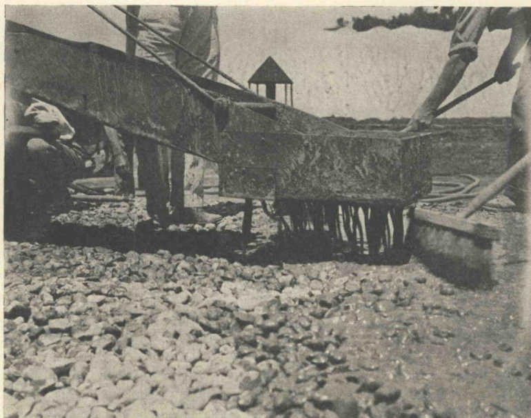
Figure 3. Grout was applied through a special distributing box on the end of the mixer spout.
