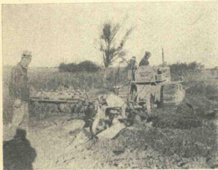
Figure 9. Fourteen-inch gang plow used in place of orchard cultivators during wet mixing. Note dry soil-cement mixture which is being turned up by the plow. Missouri photo.
