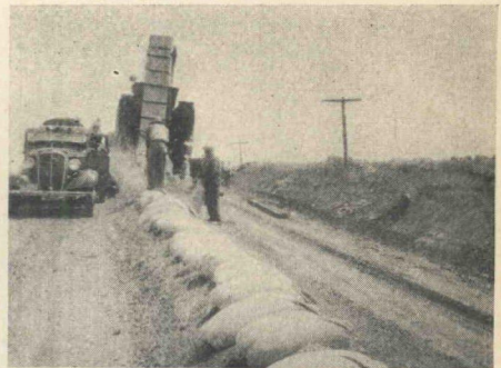
Figure 6. Sacks of cement are placed in the specified amount on top of windrow and are dumped over windrow just in advance of traveling mixing plant to prevent loss of cement by wind. Note some dusting at spiral feeders on machine. Supply truck is furnishing water for mix. Missouri photo.
