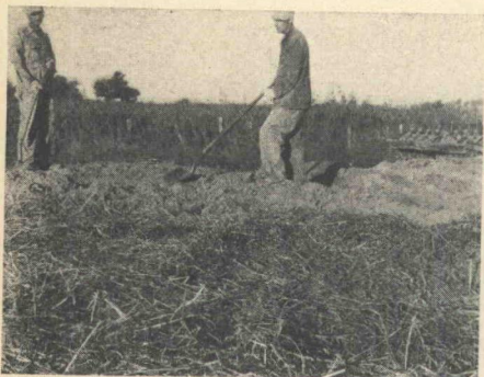
Figure 21. View showing straw placed on finished surface and covered with approximately six inches of dirt for turn-around for mixing equipment. Missouri photo.
