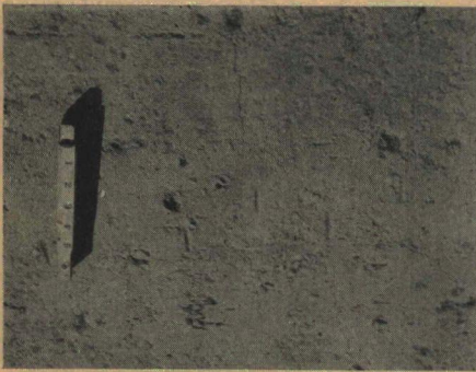
Figure 3. Close-up of surface of 8 per cent cement soil-cement mixed-in-place base after 7 days of cover with Sisalkraft paper. Note only very slight incipient cracking of surface.
