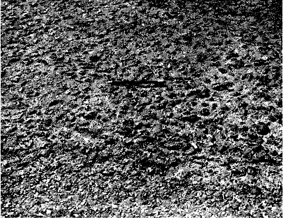
Figure 1. Rumble strip surface texture after one year, Case II, Third Street.
