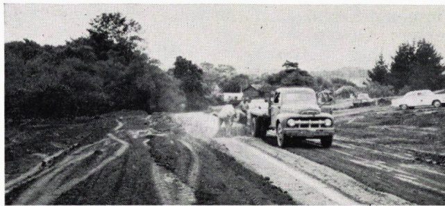
Figure 3. First known installation (July 1958) of reinforced concrete pipe with baled straw protection. Baled straw being placed directly on top of pipe after conventional granular backfill completed.
