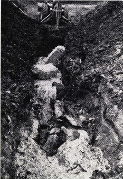
Figure 5. Trenching and straw placement above existing 36-in. R.C.P. ( D -load=1,750 lb) to be covered with 62-ft fill to convert existing expressway to full freeway. Trench cave-in will do no serious harm, even though it is desirable to maintain vertical sides. Excavation being performed in unsuitable material from previous construction project.
