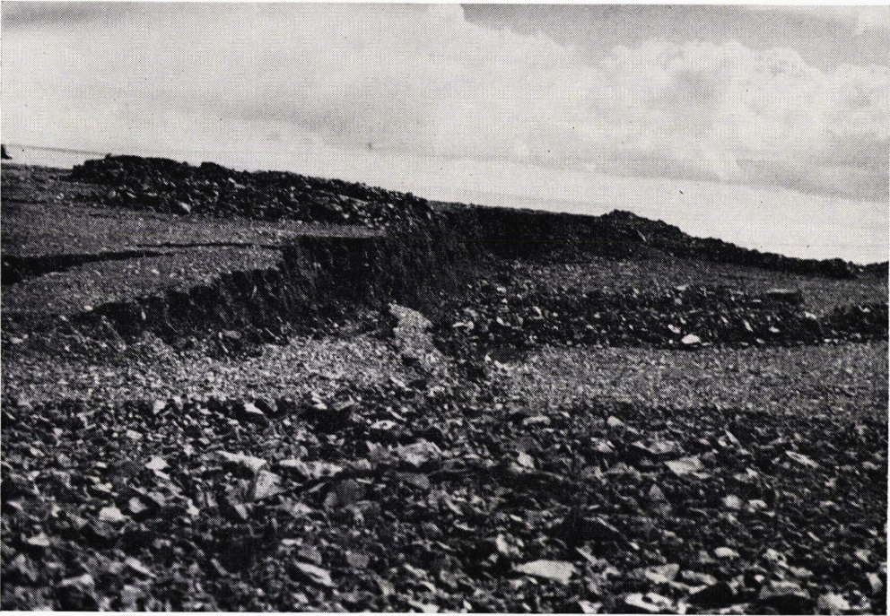
Figure 3. Nose of fill dropped about 7 ft (see Fig. 4).
