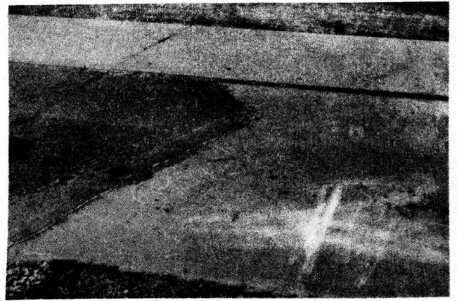
FIGURE 18. THIS IS A VIEW OF THE FIRST CRACK PAST THE JOINT IN FIGURE 17.
