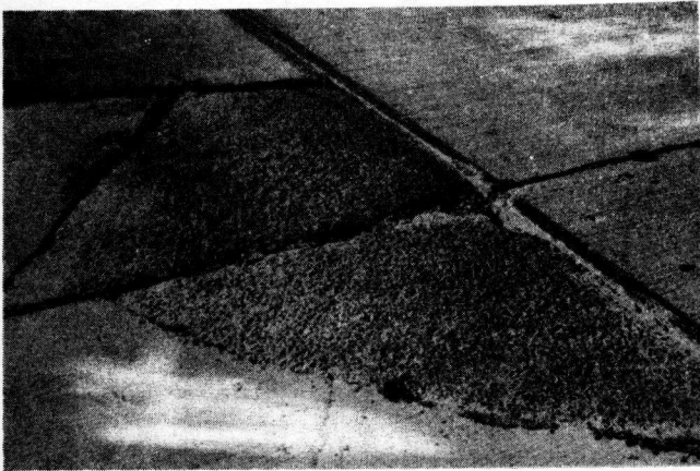
FIGURE 17. THIS SLAB TREATED WITH MIX "B" HAD FAILED DUE TO AN EQUIPMENT FAILURE DURING TREATMENT.
