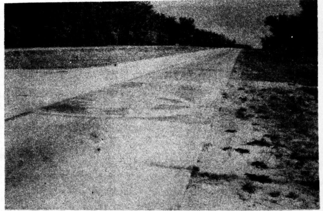
FIGURE 8. VIEW OF THE PATCH ON THE SAME SLAB (FIGURE 7) IN NOVEMBER, 1944. PUMPING IS STILL SEVERE.
