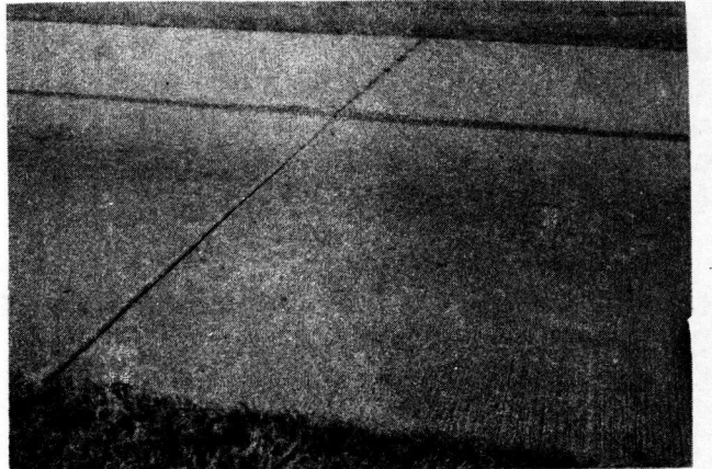
FIGURE 16. AN UNTREATED SLAB (IN THE AREA IN WHICH THE JOINTS WERE TREATED WITH MIX "B") THAT HAD SETTLED \frac{3}{4} OF AN INCH.
