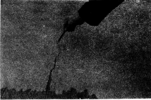
FIGURE 11. FIRST STAGES OF CRACKING DUE TO SLAB PUMPING.
