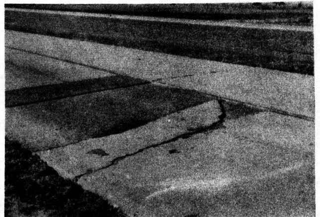
FIGURE 20. THE JOINT AT STATION 662+46 (ADJACENT TO SLAB IN FIG. 19 WAS NOT TREATED AND HAS GIVEN TWO YEARS OF UNSATISFACTORY PERFORMANCE.
