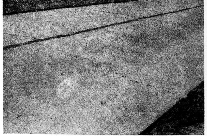
FIGURE 12. ADVANCED STAGES OF CRACKING IN WHICH SPALLING OCCURS CAUSED BY SEVERE SLAB MOVEMENT.
