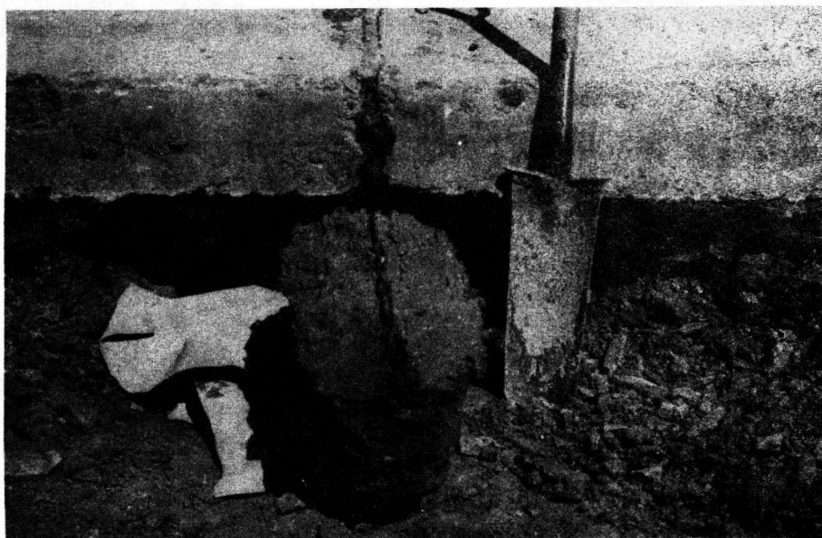
FIGURE 2. UNDISTURBED COLUMN OF SOIL REMOVED FROM UNDER A PUMPING EXPANSION JOINT. NOTE THAT A SOFT MUD HAD FORMED ONLY UNDER THE FAR SIDE OF THE JOINT IN THE DIRECTION OF TRAFFIC.
