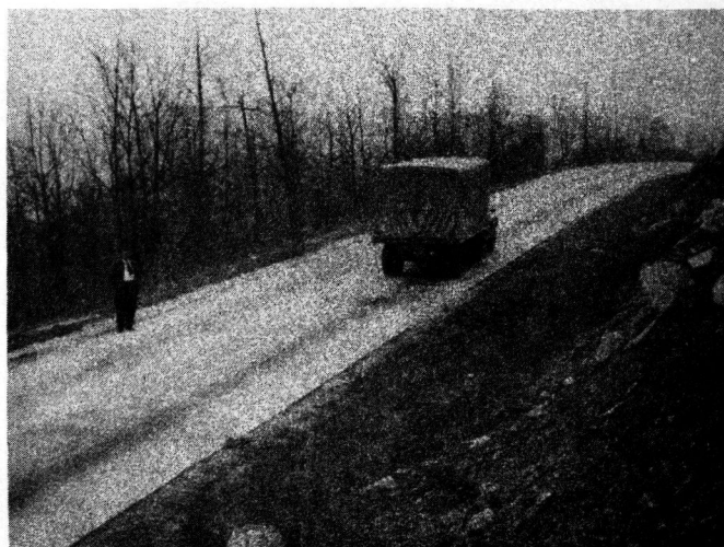
FIGURE 4. ANOTHER EXAMPLE SHOWING THE DIFFERENCE IN THE OIL STREAKS IN THE UP-HILL AND DOWNHILL LANES DUE TO SPEED OF TRAFFIC ON A LONG 6% GRADE. NOTE THE PUMPING AND DAMAGE TO PAVEMENT IN THE UPHILL TRAFFIC LANE. FAP 269 B MARION COUNTY (3-22-44)
