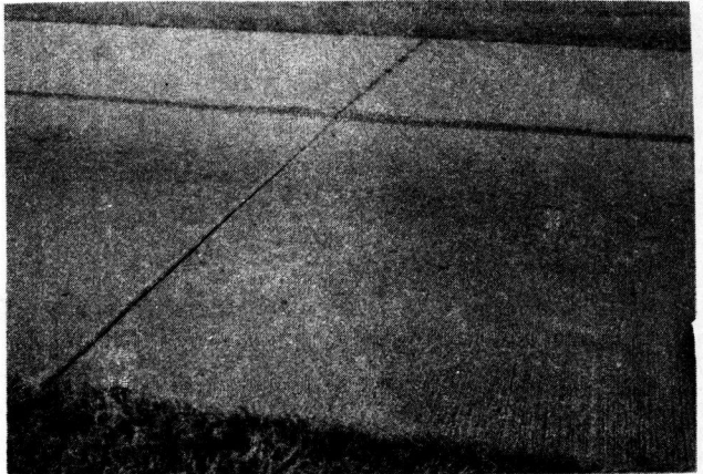
FIGURE 16. AN UNTREATED SLAB (IN THE AREA IN WHICH THE JOINTS WERE TREATED WITH MIX "B") THAT HAD SETTLED \frac{3}{4} OF AN INCH.
