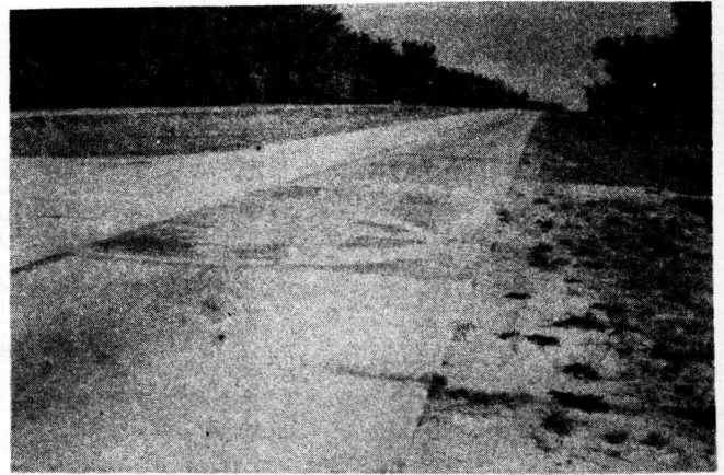
FIGURE 8. VIEW OF THE PATCH ON THE SAME SLAB (FIGURE 7) IN NOVEMBER, 1944. PUMPING IS STILL SEVERE.
