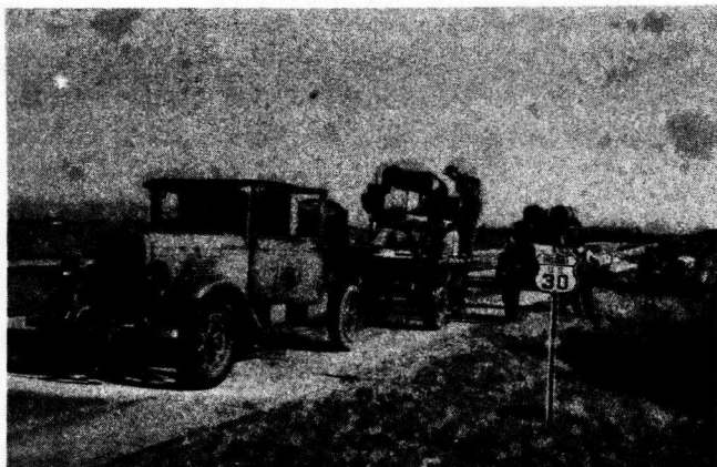
FIGURE 2. MUD-JACKING EQUIPMENT - AIR COMPRESSOR, MUD-JACK, WATER TANK MIXER, TAR KETTLE, AND SUPPLY TRUCK.
