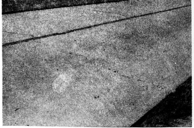
FIGURE 12. ADVANCED STAGES OF CRACKING IN WHICH SPALLING OCCURS CAUSED BY SEVERE SLAB MOVEMENT.
