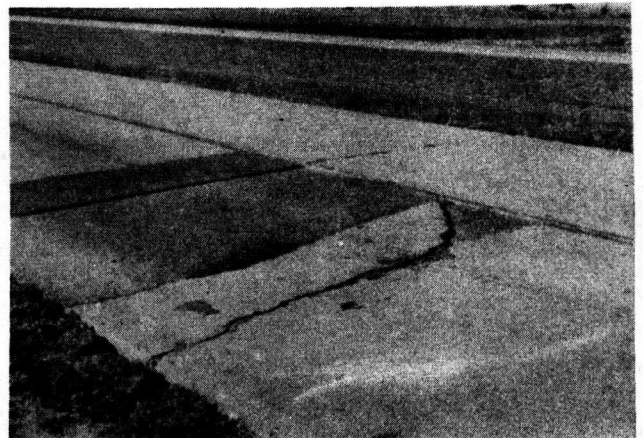
FIGURE 20. THE JOINT AT STATION 662+46 (ADJACENT TO SLAB IN FIG. 19 WAS NOT TREATED AND HAS GIVEN TWO YEARS OF UNSATISFACTORY PERFORMANCE.
