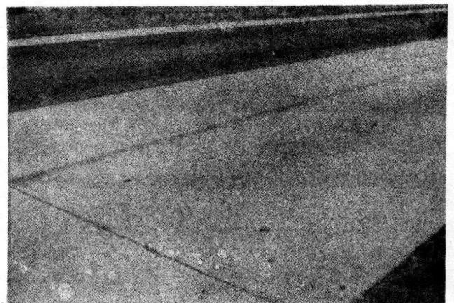
FIGURE 22. THIS JOINT, TREATED WITH MIX "D", PERFORMED SATISFACTORILY DURING TWO YEARS OF SERVICE.
