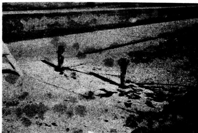
FIGURE 4. THE HOLES WERE PLUGGED TO PREVENT THE SLAB FROM SETTLING AND SQUEEZING OUT THE MIX UPON COMPLETION OF MUD-JACKING.
