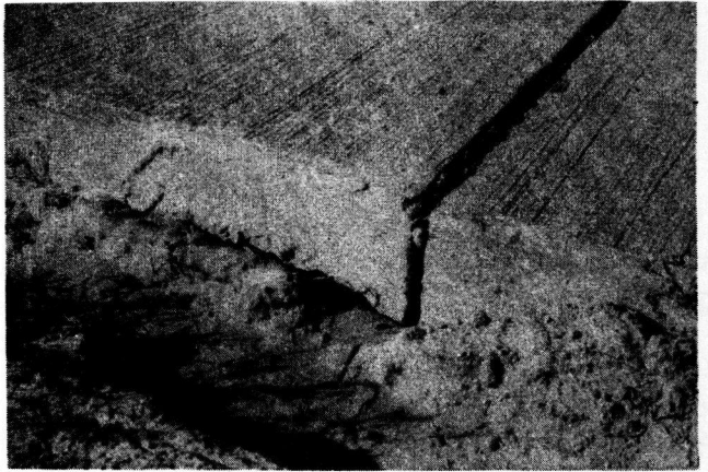
FIGURE 14. SEVERE PUMPING AT AN UNTREATED JOINT IN THE SECTION OF PAVEMENT IN WHICH JOINTS WERE TREATED WITH MIX "A"
