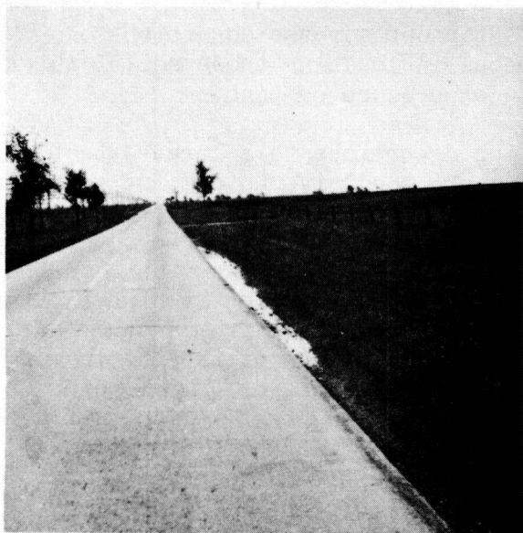
Figure 8. Water trapped at the pavement edge fosters pumping. The joints and cracks opposite the water in the picture are pumping.
