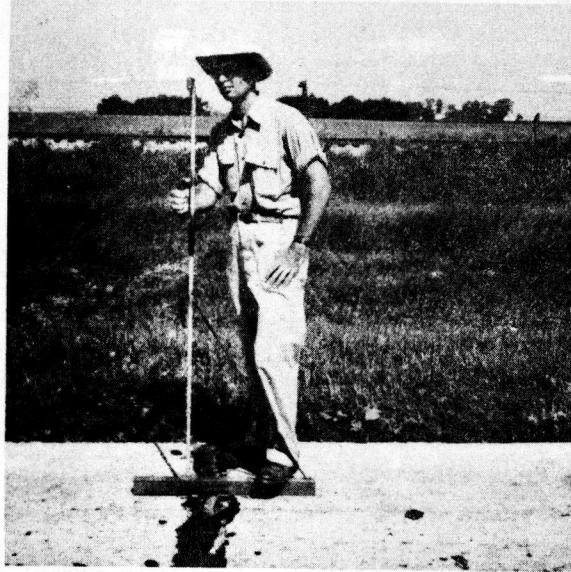
Figure 4. Measurement of depth of fault being made with device which permits readings at eye level.
