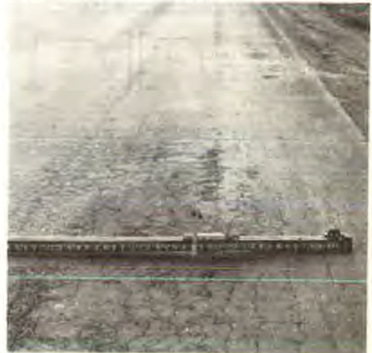
Figure 3. Class "B" failure.
