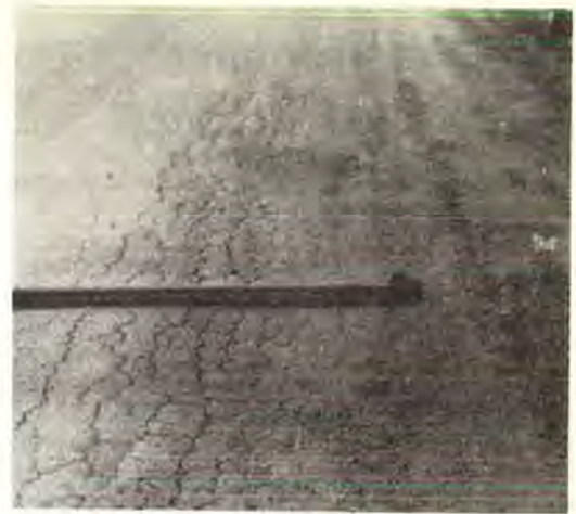
Figure 2. Class "A" failure.
