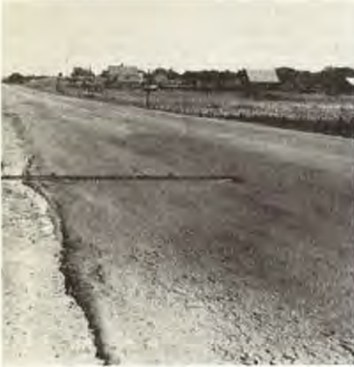
Figure 4. Class "C" failure.
