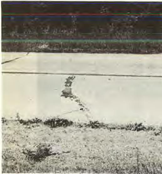
Figure 8. Irregular transverse cracking in east lane of Section 5-R in May 1949. Section does not contain wire mesh reinforcement.
