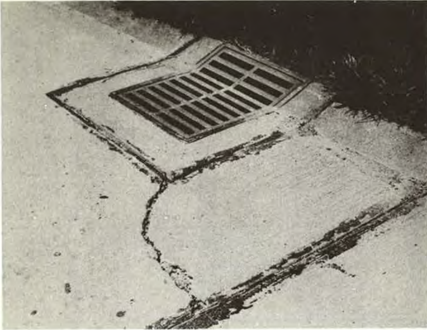
Figure 6. Typical of cracking where drop inlet is constructed near joint installation, Section 4-R in May 1949.
