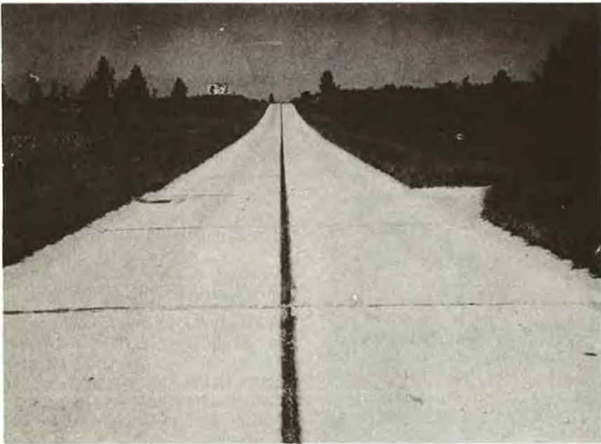
Figure 7. Faulted joint in foreground, Section 4-R. Pavement contained expansion joints at 120 foot spacing with dowel bars and contraction joints at 20 feet without dowel bars. Wire mesh reinforcement was not installed in this section.
