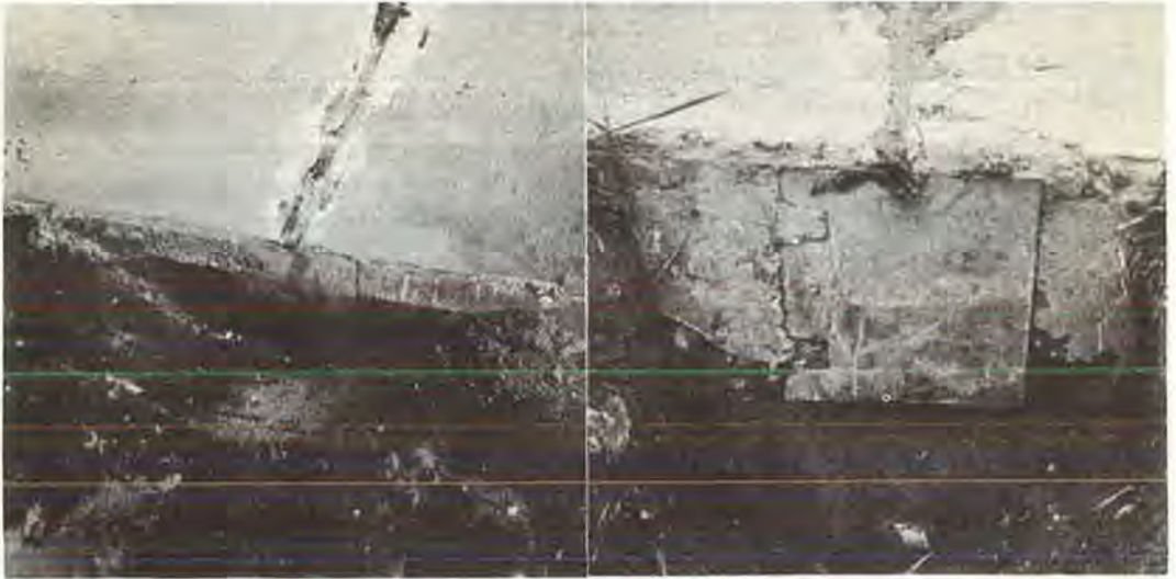
Figure 28. Air chamber expansion joint, Type DB-1 (3) Series 5, Station 79+60. (Left) at time of construction, 1940. (Right) 10 years later, 1950.
