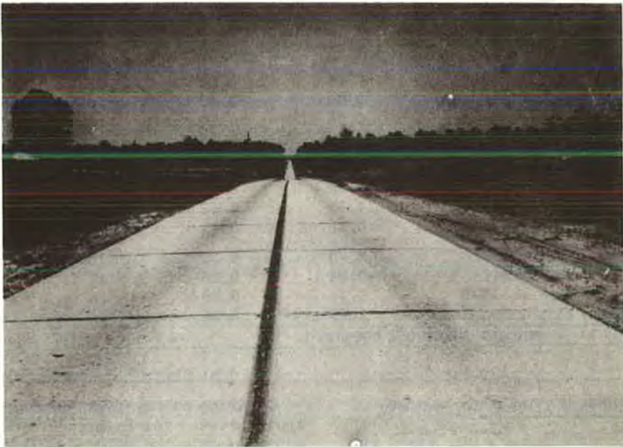
Figure 5. View to north of Section 2-R through Section 1 in May 1949. Pavement in foreground contains expansion joints at 800 foot intervals with dowel bars and contraction joints at 200 foot intervals without dowel bars. Wire mesh reinforcement was not used in this section.
