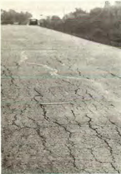
Figure 1. Cracking of concrete pavement in Georgia.
