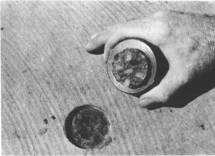
Figure 11. Typical cohesive bond failure in concrete.
