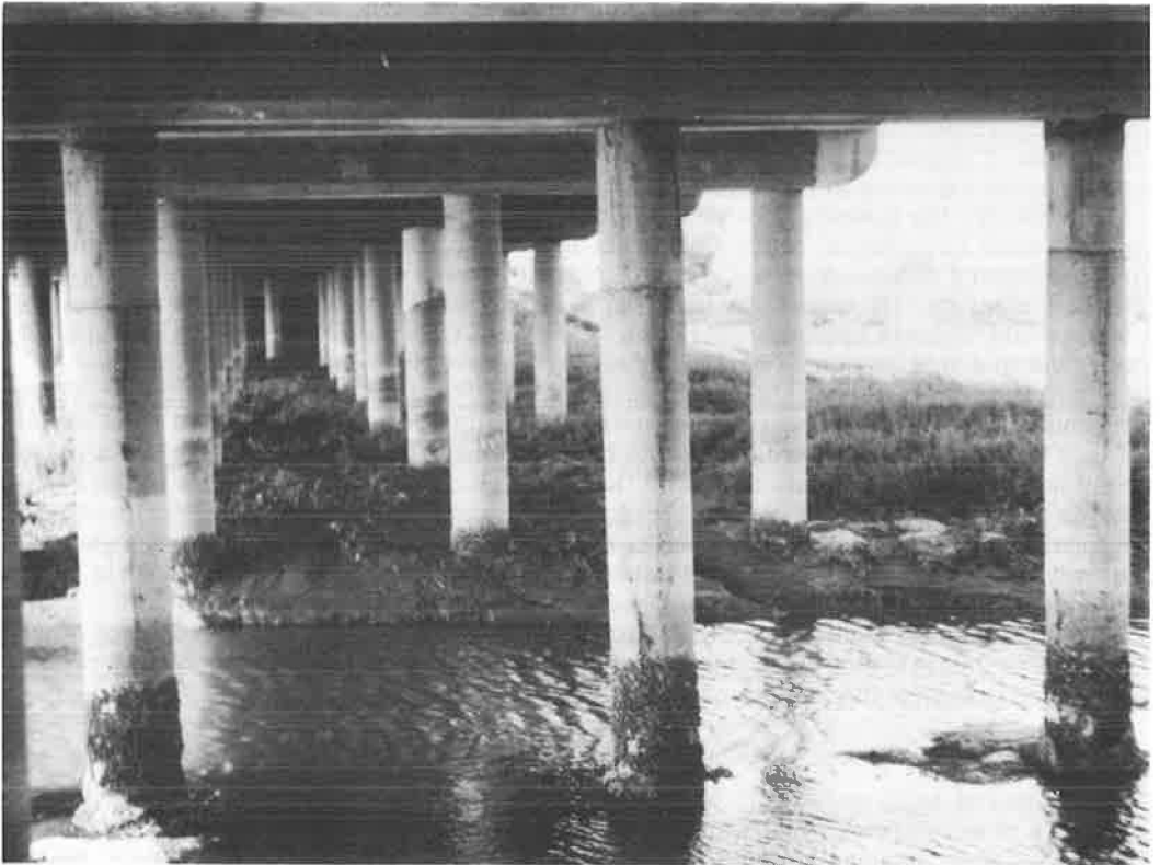
Figure 1. Vertical concrete cracking of 10-yr-old reinforced concrete bridge piles in tidal water near San Diego, Calif., 1962.
