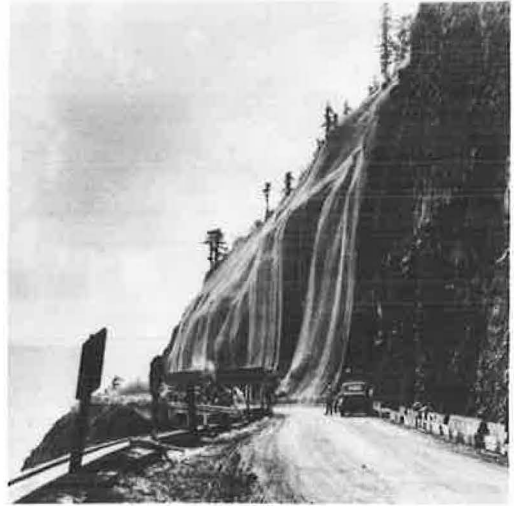
Figure 5. Wire netting, rockfall area on old construction.
