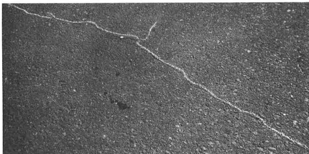
Figure 30. Shrinkage crack between the two test strips (Fig. 29).
