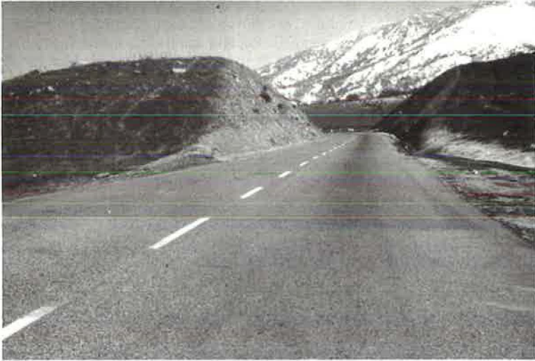
Figure 26. White Wolf Grade section six months after treatment: treated lanes in background; untreated lanes in foreground.
