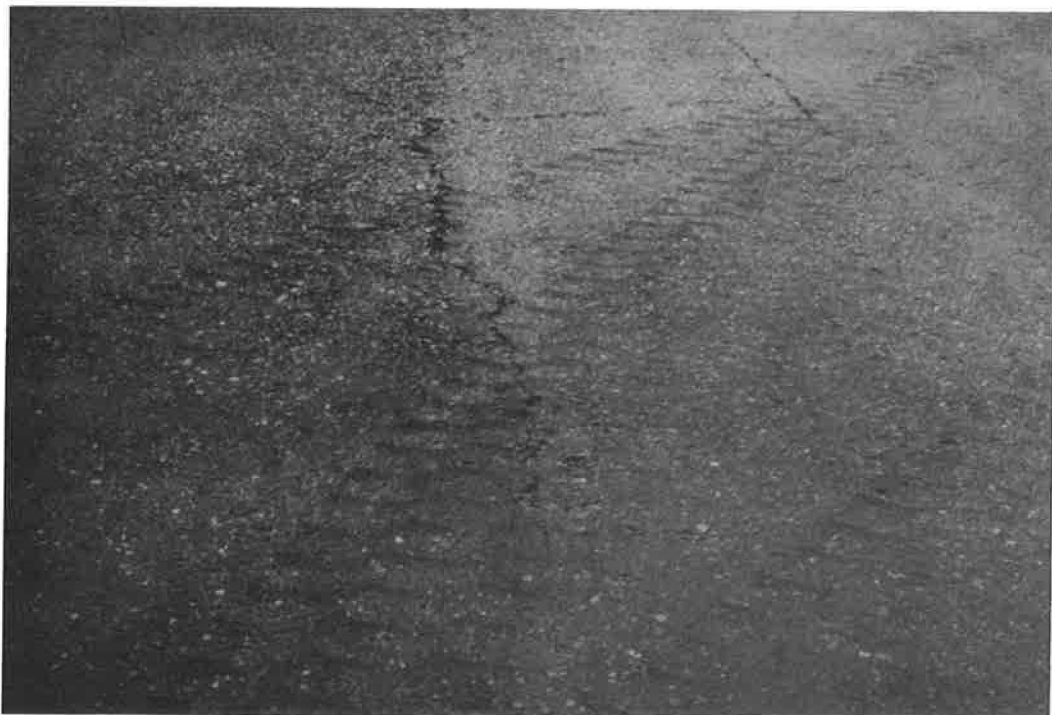
Figure 25. Taxiway at Edwards AFB viewed from treated area toward untreated control section.
