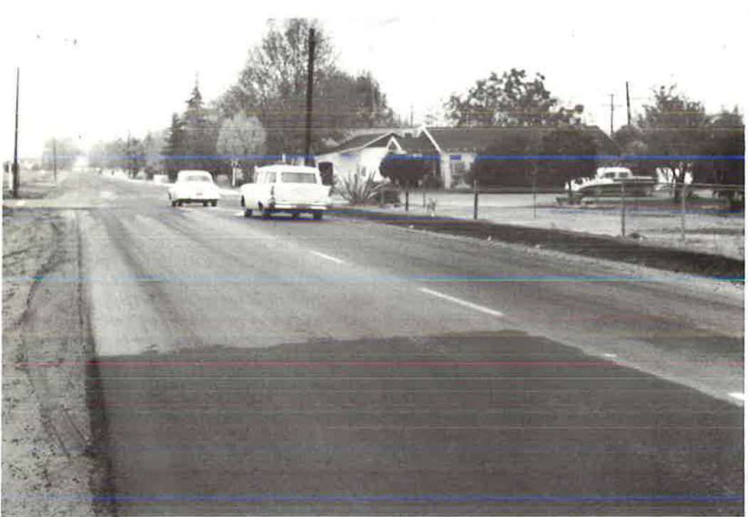
Figure 22. Asphalt section treated with cationic maltene emulsion as construction seal: after rainstorm treated section dried quickly (background); untreated portion retains water in pores (foreground).
