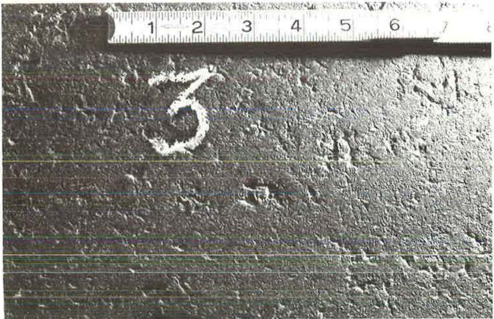
Figure 10. Variations in surface texture, North 13th Street, Manville, N. J., asbestos mix with 8 to 9.5 percent asphalt content.
