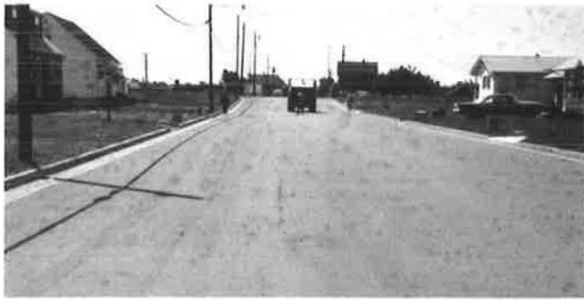
Figure 13. Joint crack in standard pavement stopping at south end of asbestos pavement, North 13th Street, Manville, N. J., July 1962.
