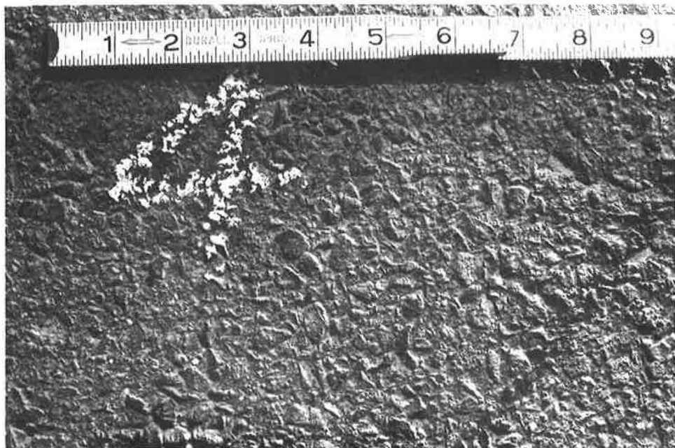
Figure 9. Variations in surface disintegration, North 13th Street, Manville, N. J., August 1962, standard pavement mix.
