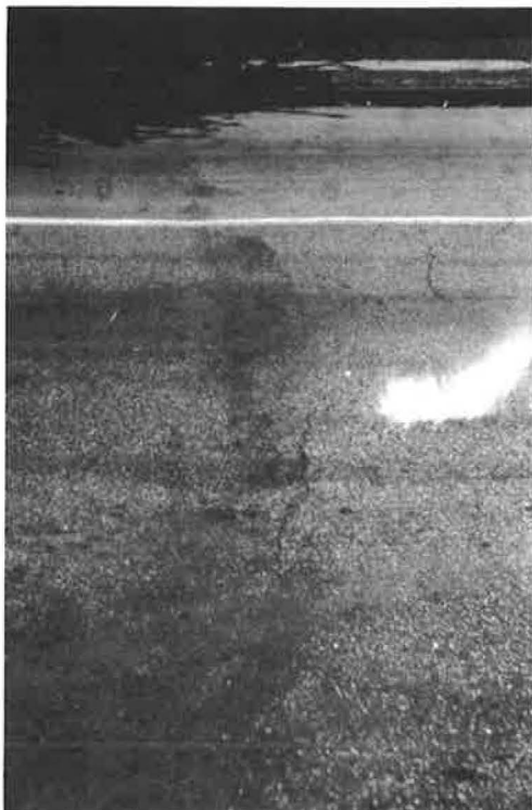
Figure 15. Reflection cracking, Ross Avenue, Dallas, Texas, August 1962.
