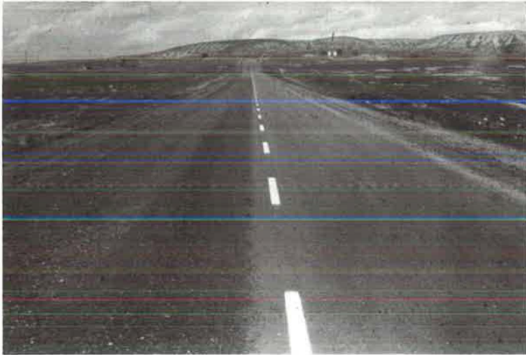
Figure 27. Weathering of road mix more rapid than for asphalt concrete accounting for contrast in surface texture nine months after application: treated lane, right; untreated lane, left.
