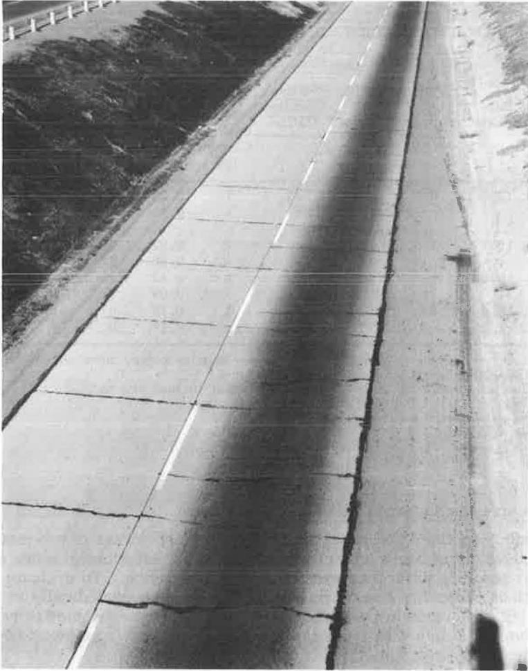
Figure 14. Pavement containing \text{CaCl}_2 , Merced County.
