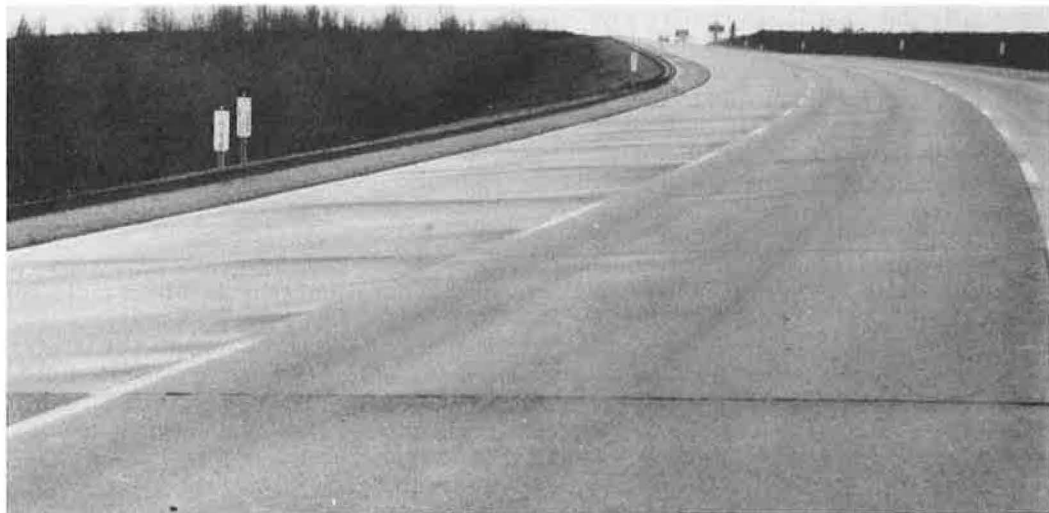
Figure 11. Curled pavement slabs.
