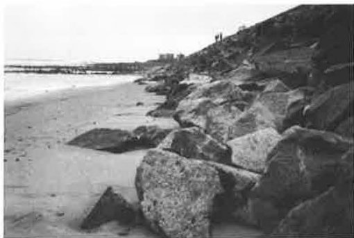
Figure 6. Displaced stones after severe storms.
