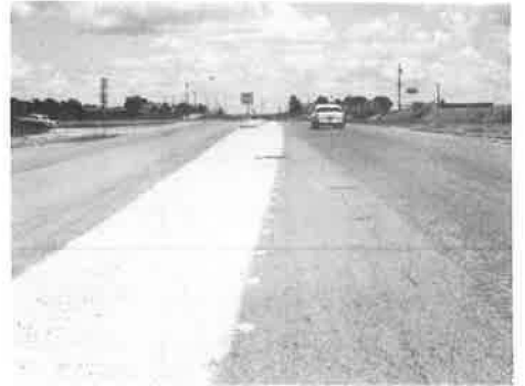
CONDITION 3 - RUMBLE STRIP
