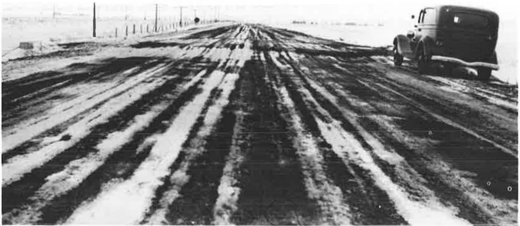
Figure 11. Combination culvert heave and fill shrinkage causing dangerous bump (northern Minn.).
