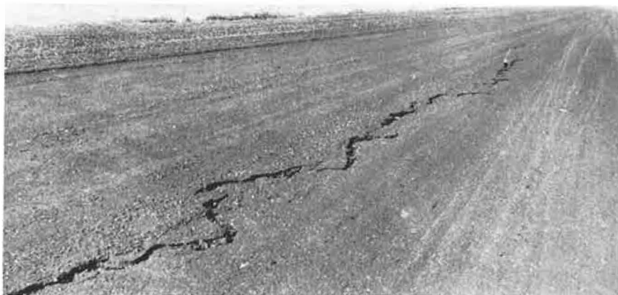
Figure 7. Large crack caused by shrinkage of dense clay subgrade following deep frost penetration (Minn.).
