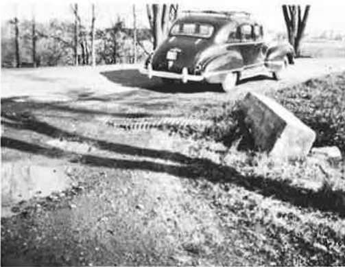
Figure 17. Headwall shoved from original position.
