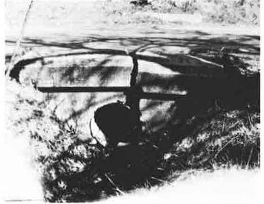
Figure 16. Concrete headwall cracked by differential heaving.
