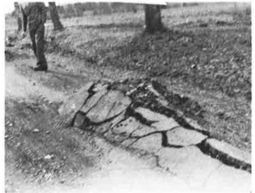
Figure 20. Damage caused by excessively heavy traffic.
