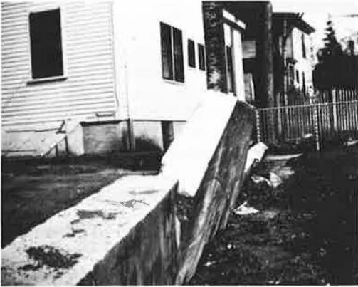
Figure 15. Low retaining wall thrown out of position because of freezing.
