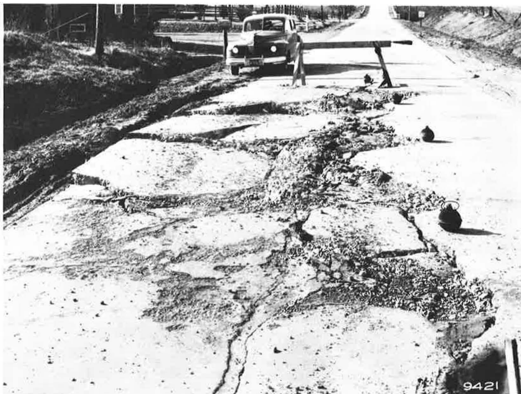
Figure 5. Extreme example of pavement damage resulting from frost action.
