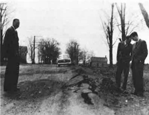
Figure 19. Damage caused by excessively heavy traffic.
