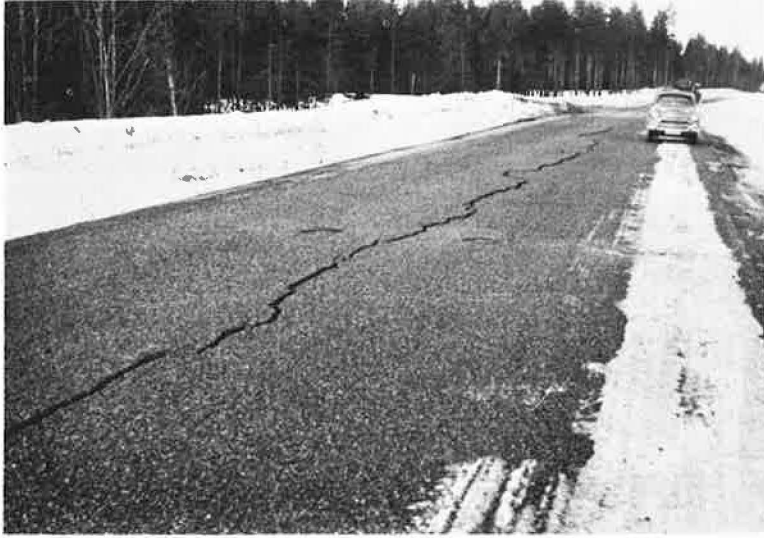
Figure 6. Frost crack in a road near Ersnäs.
