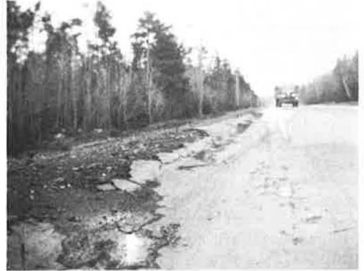
Figure 18. Shoulder elevated above pavement proper.
