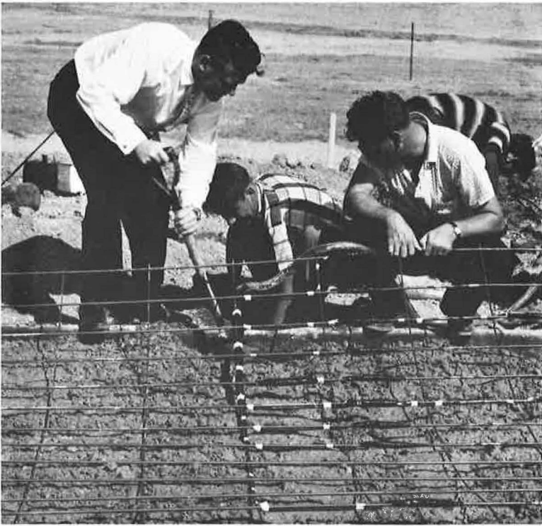
Figure 3. Welded-wire reinforcing steel mesh with SR-4 strain gages bonded to longitudinal steel being installed.
