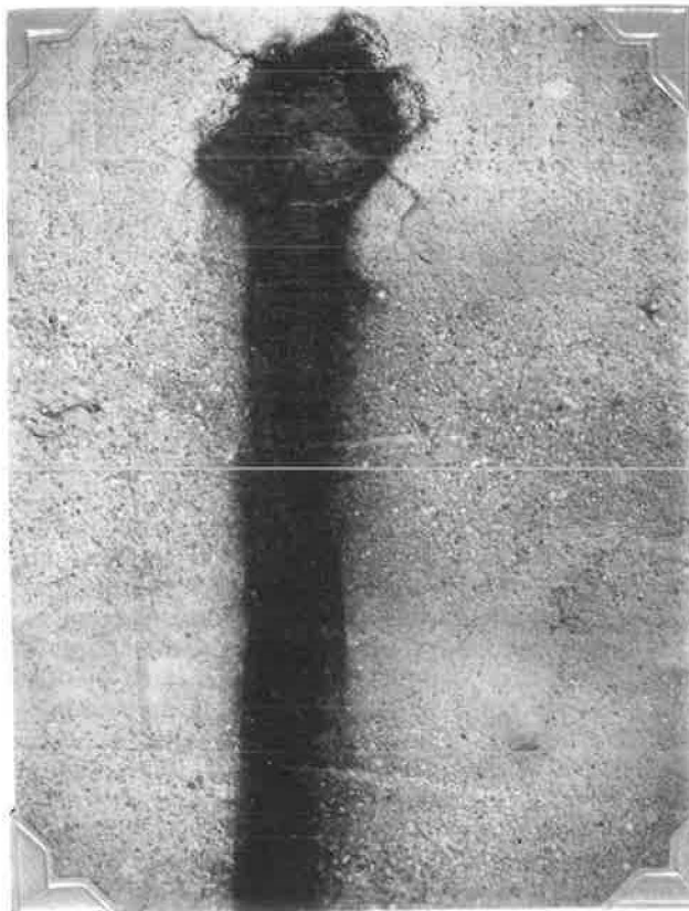
Figure 2. Surface of concrete retaining wall displaying staining and surface pitting produced by oxidation and hydration of pyrite in a particle of coarse aggregate. Magnification \times \frac{1}{4} . (Courtesy of the Ohio Department of Highways.)
