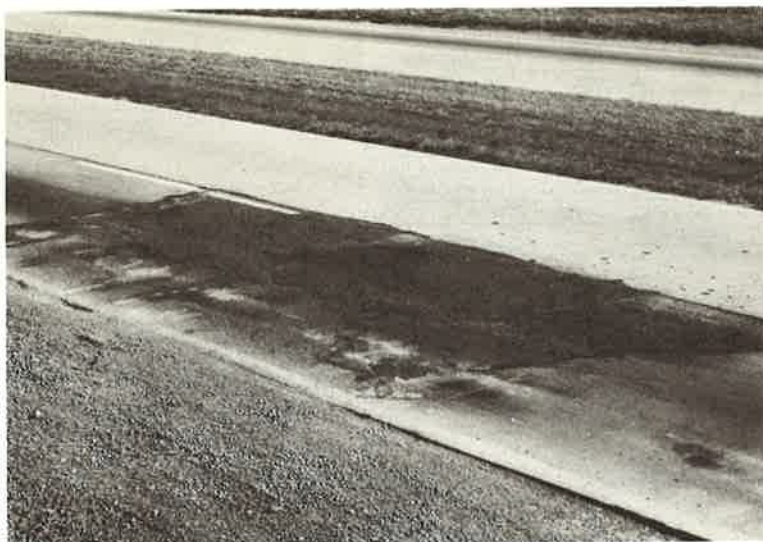
Figure 6. Failure in 7-in. pavement, Hamburg.
