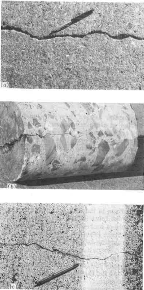
Figure 3. Typical crack on York pavement: (a) spalled appearance at surface, (b) core removed directly over crack, (c) appearance of crack at edge of pavement.
