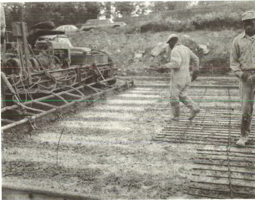
Figure 8. Pavement construction showing internal vibration of concrete, and staggered ends of bar mats.
