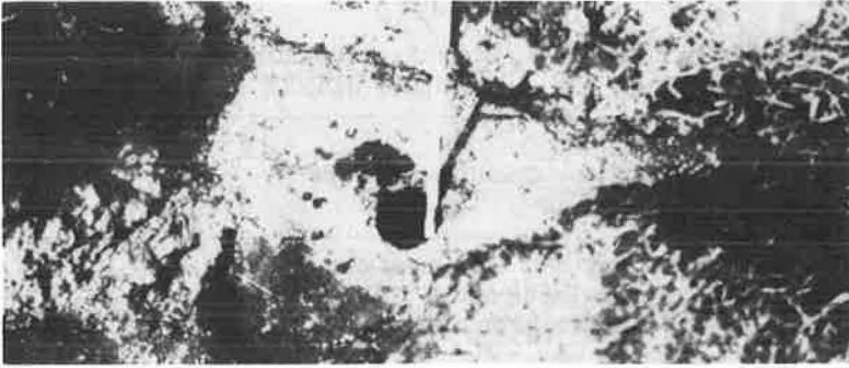
Figure 11. Crack and test pit, membrane peeled back from embankment, Str. 13, summer 1952.
