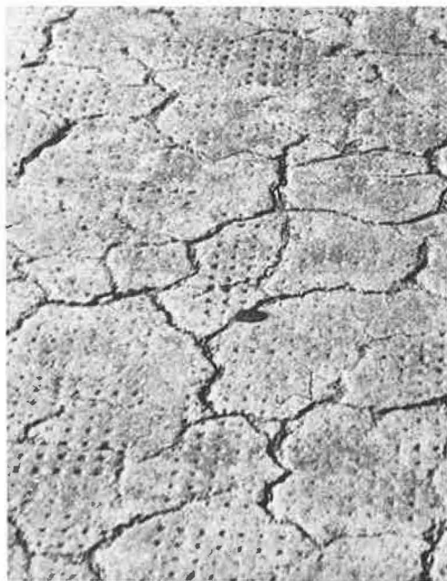
Figure 3. Typical pattern cracking in sidewalk in Kingston.
