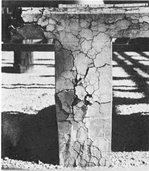
Figure 1. Deteriorated concrete with Gull River carbonate rock as coarse aggregate.
