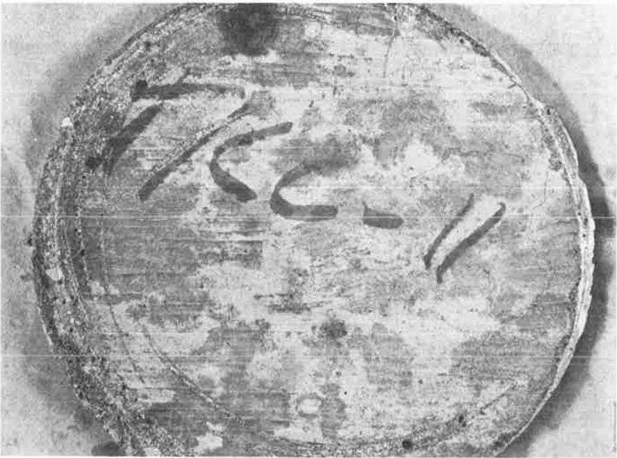
Figure 20. KC-11, finished wall surface, three-quarter size. Mottled appearance of surface is due to poor bond between wood-formed surface and rubbed on cement paste. Light areas are rubbed cement still adhering to original surface. Impression of wood form is apparent. Irregular dark lines are penciled traces of fine shrinkage cracks.
