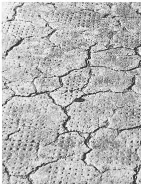
Figure 3. Typical pattern cracking in sidewalk in Kingston.
