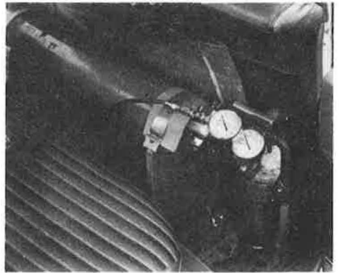
Typical Nitrogen Bottle Installation - Used With FM 200.
