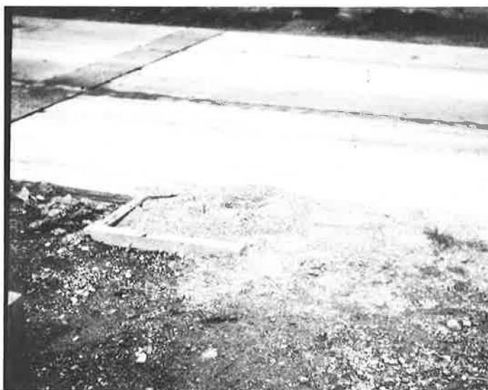
Figure 12. Pumping at U-5, L-5—Oct. 30, 1962.
