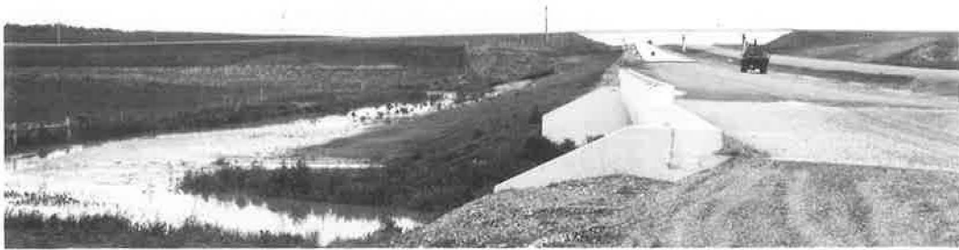
Figure 3. Water standing in poorly drained channel between sections.
