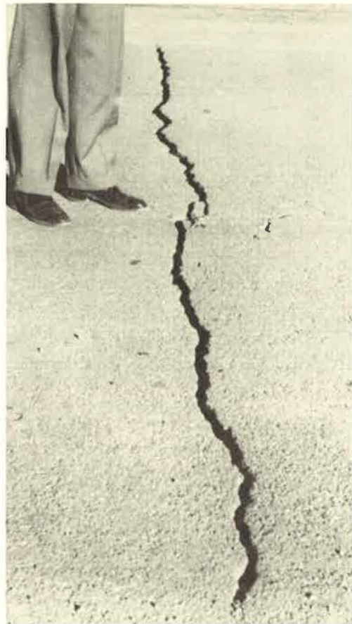
Figure 15. Transverse cracks ranging from \frac{3}{4} to 1\frac{1}{2} in. in width.
