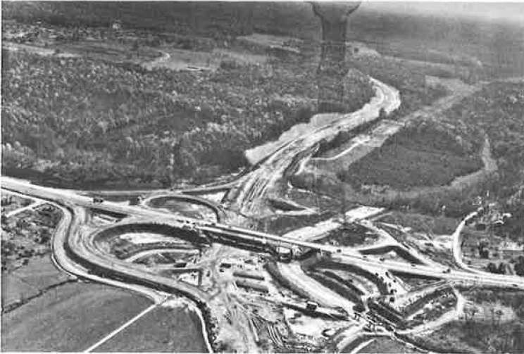
Figure 2. Interchange of Route 236 and Capital Beltway under construction in November 1959, showing large vacant tract in upper left.
