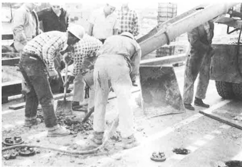
Figure 4. Pouring intermediate diaphragm within cells of prototype structure between Phases II and III.
